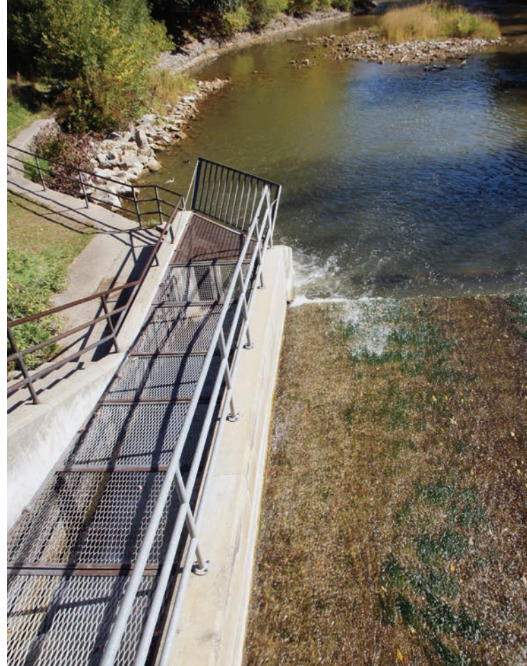
▲ The fish ladder on the left is covered by a grill to protect salmon using the steps.
